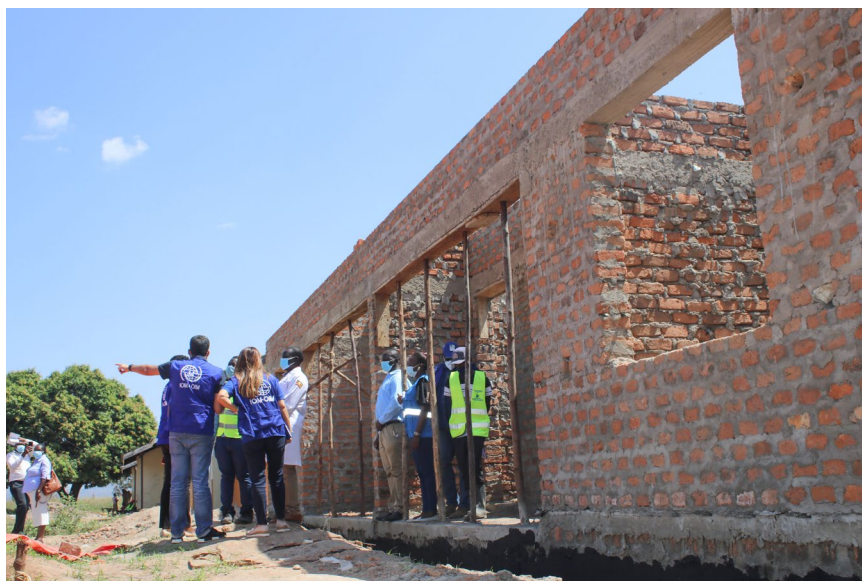
IOM, Ministry of Health and Amuru District local government inspect the construction works recently ©IOM
