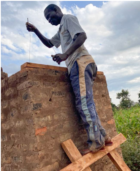
Peter Mackuel constructing a latrine for fellow refugees in the Kiryandongo Refugee Settlement ©UNHCR Uganda
