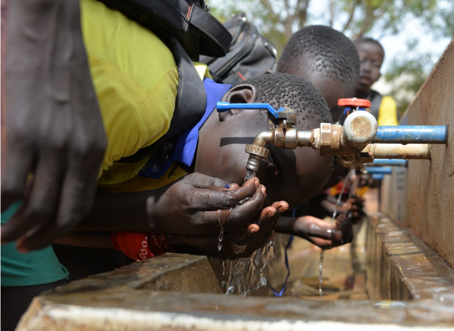
Pupils of Nyumazi Primary school in Adjumani district drink clean and safe water from taps in the school compound. The water is pumped from the solar powered system constructed under the Water, Sanitation and Hygiene (WASH) project with funding from the Government of the Republic of Iceland ©UNICEF Uganda
