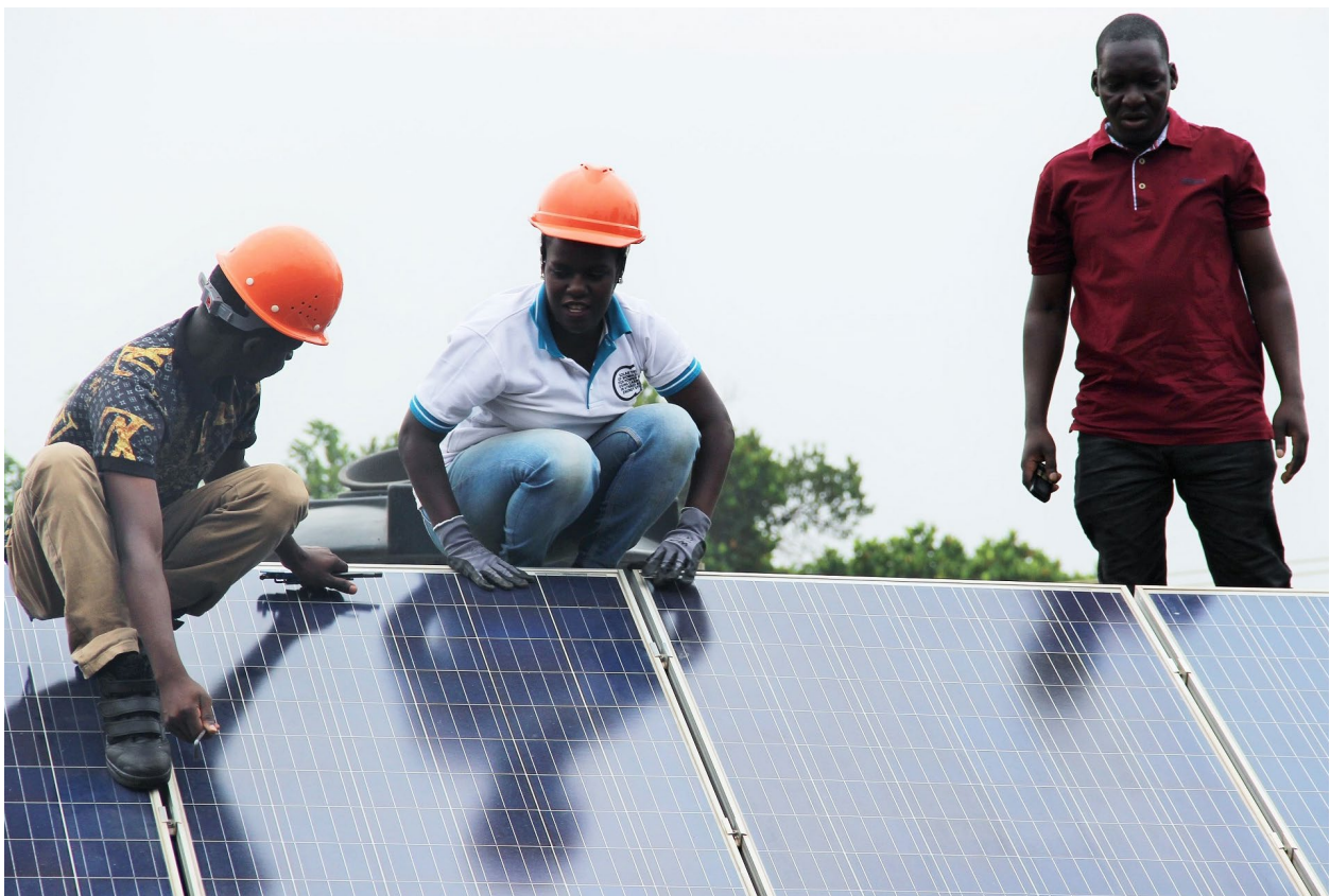
Ms. Afuswa Karungi, a graduate volunteer, with technicians from Green Heat Uganda Limited install solar panels ©UNDP
