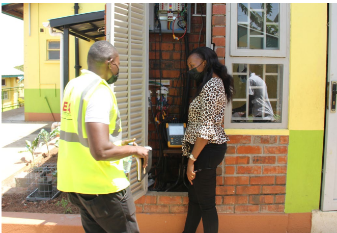
UNDP and Uganda Electricity Regulatory Authority (ERA) staff inspect the newly installed electrical system at Mwanamugimu Nutrition Unit in Uganda's National Referral (Mulago) Hospital ©UNDP Uganda
