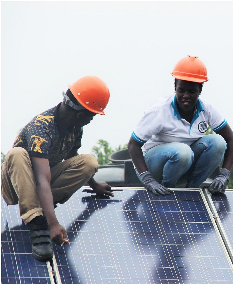
Ms. Afuswa Karungi, a graduate volunteer, with technicians from Green Heat Uganda Limited install solar panels
