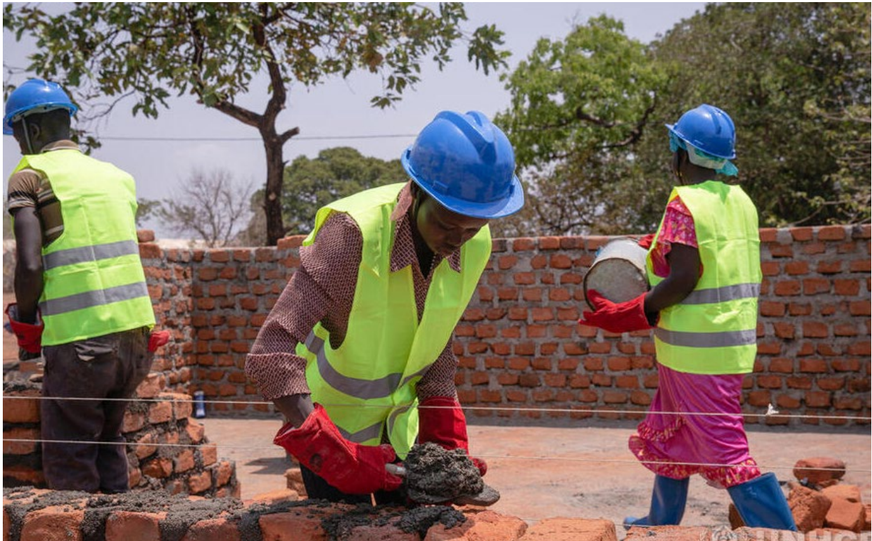
South Sudanese constructing a building in Bidi bidi Settlement, West Nile Sub-region. ©UNHCR
